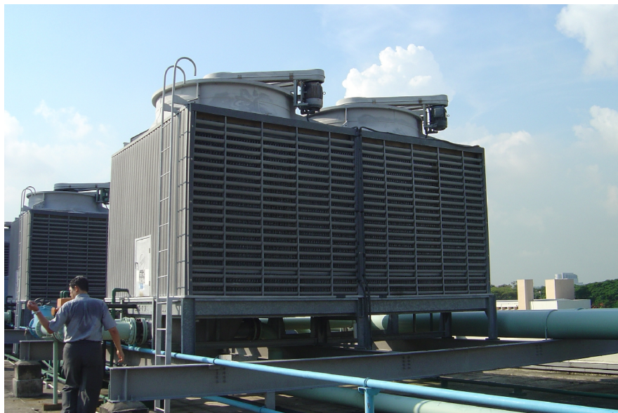
Figure 1 The photo shows the Cooling Towers of the Singapore Polytechnic
