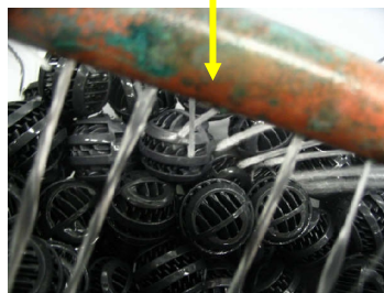
Figure 21 sprinkler close up
