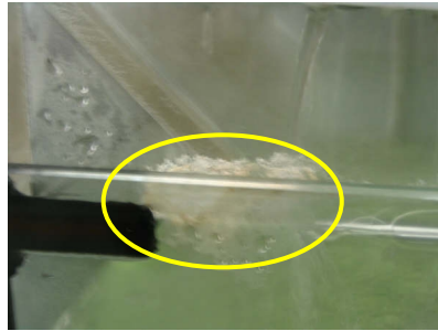
Figure 26 White stains were formed on the gaps between the water tank and the acrylic box
